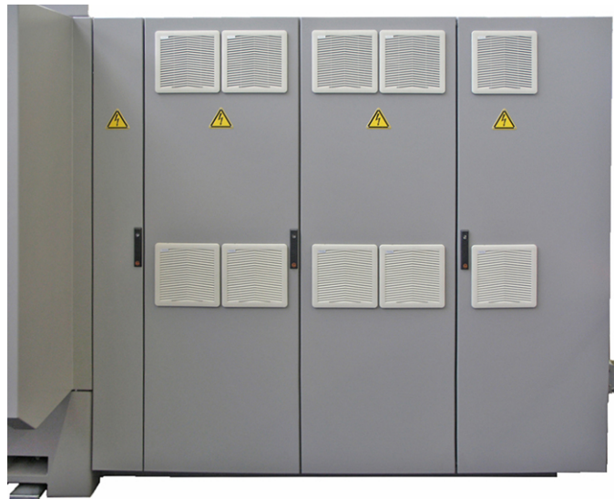
Example: Filter on the control cabinet
